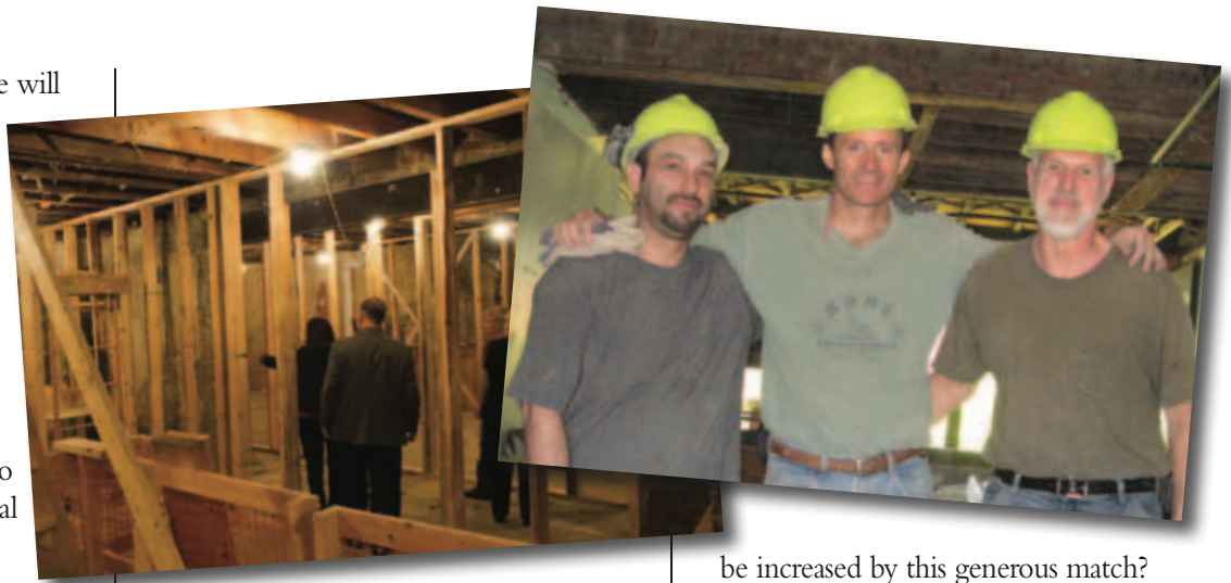
Far Left: anticipated first floor design; above: Bob Seemar (right) & workers at the building
